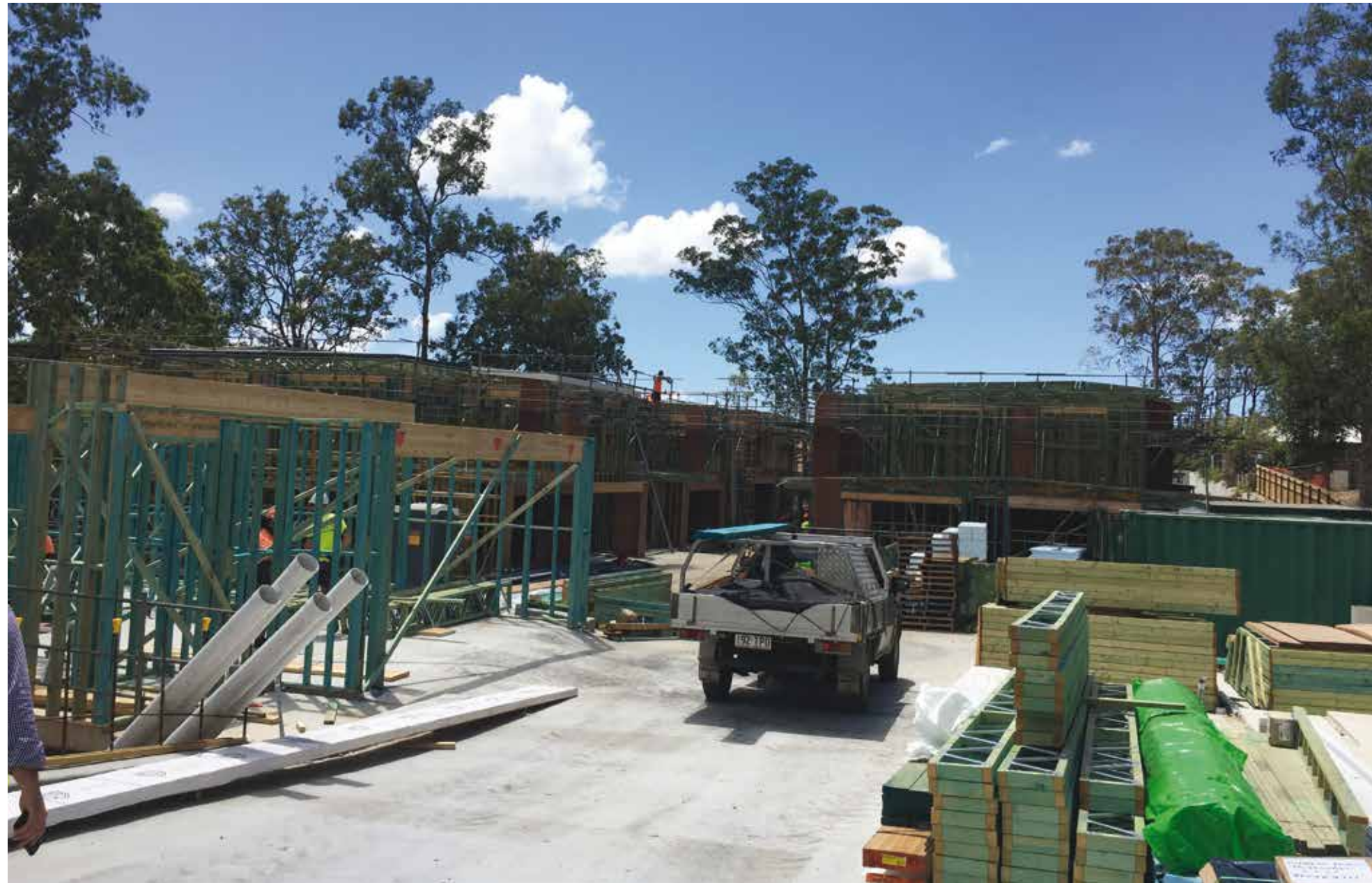
Timber flooring and wall framing, as well as the installation of roof trusses and roof sheeting were completed on town houses 3 – 7. In town houses 8 – 11, building pads were cut, ready for footings and slabs to be poured.
