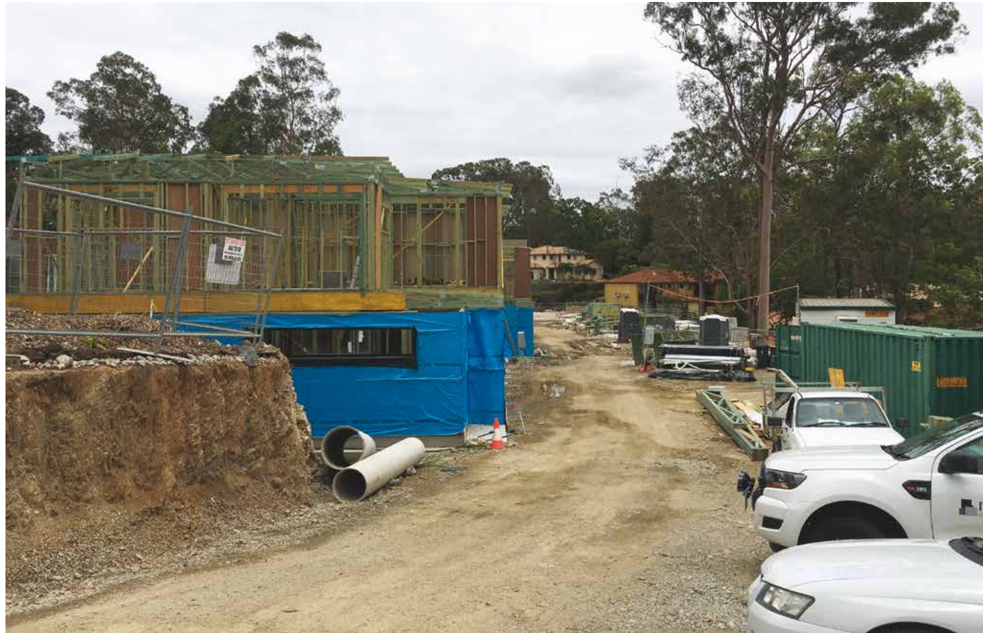
The formwork deck required for the construction of the suspended driveway entrance from Ponti Street was erected, allowing reinforcement to be tied and fixed into position to give the suspended driveway slab the necessary support.
