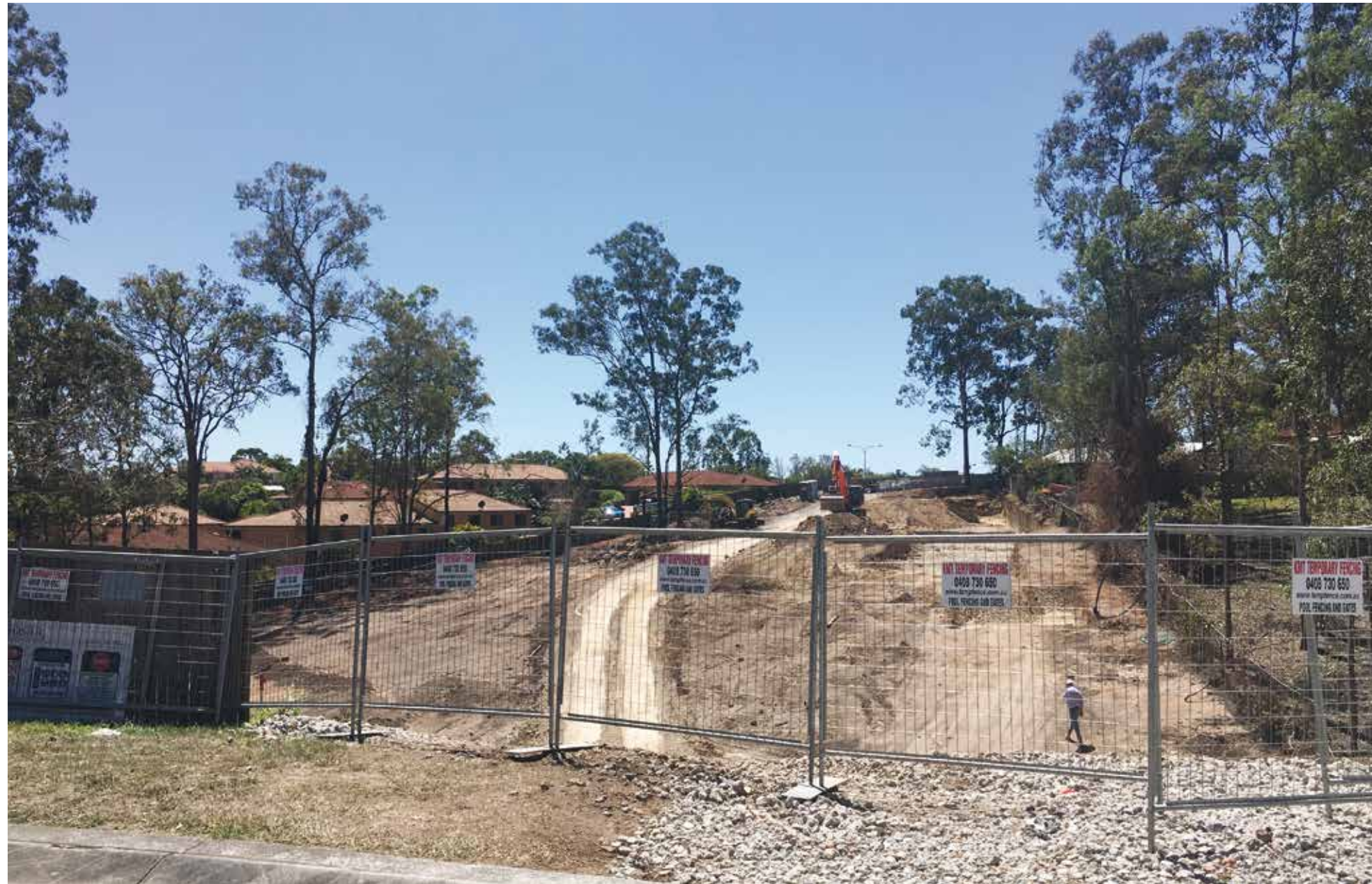
Secure perimeter fencing is now in place and existing structures have been demolished and removed from site. With the site successfully cleared, the Mosaic Construction team wasted no time, with bulk earthworks now well underway.
