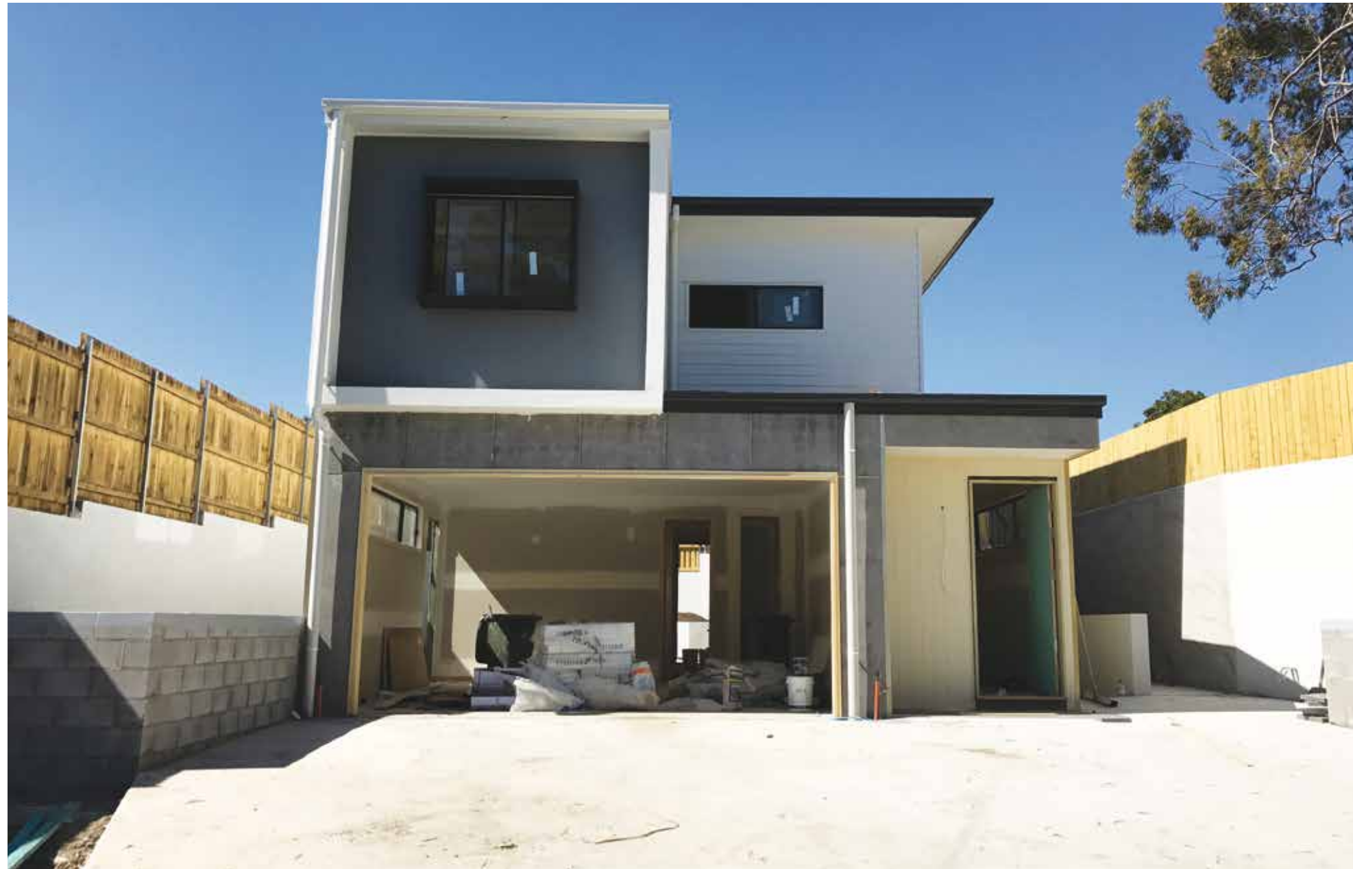
External painting is underway on town houses 1, 2 and 22 together with internal sheeting, while kitchen cabinetry, flooring and tiling commenced in town houses 3 – 7. Town houses 12 – 21 had the fixtures and lighting installed and electrical fit-off completed.
