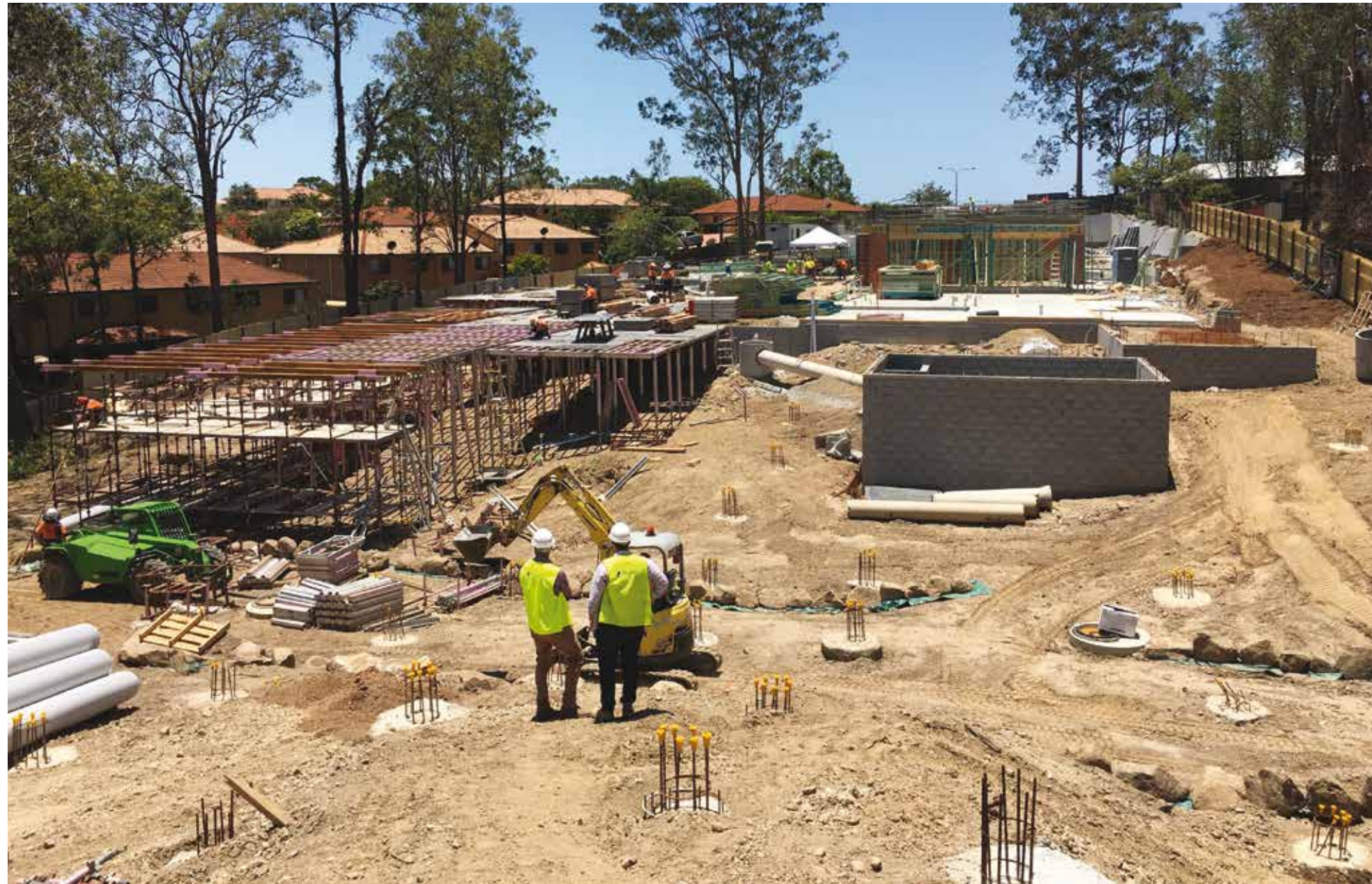
Once the detailed excavation was completed, underslab services were installed, reinforcement fixed and concrete was pumped to finish the slab. External ground floor framing is nearly complete, while the suspended timber floors were constructed and fixed.
