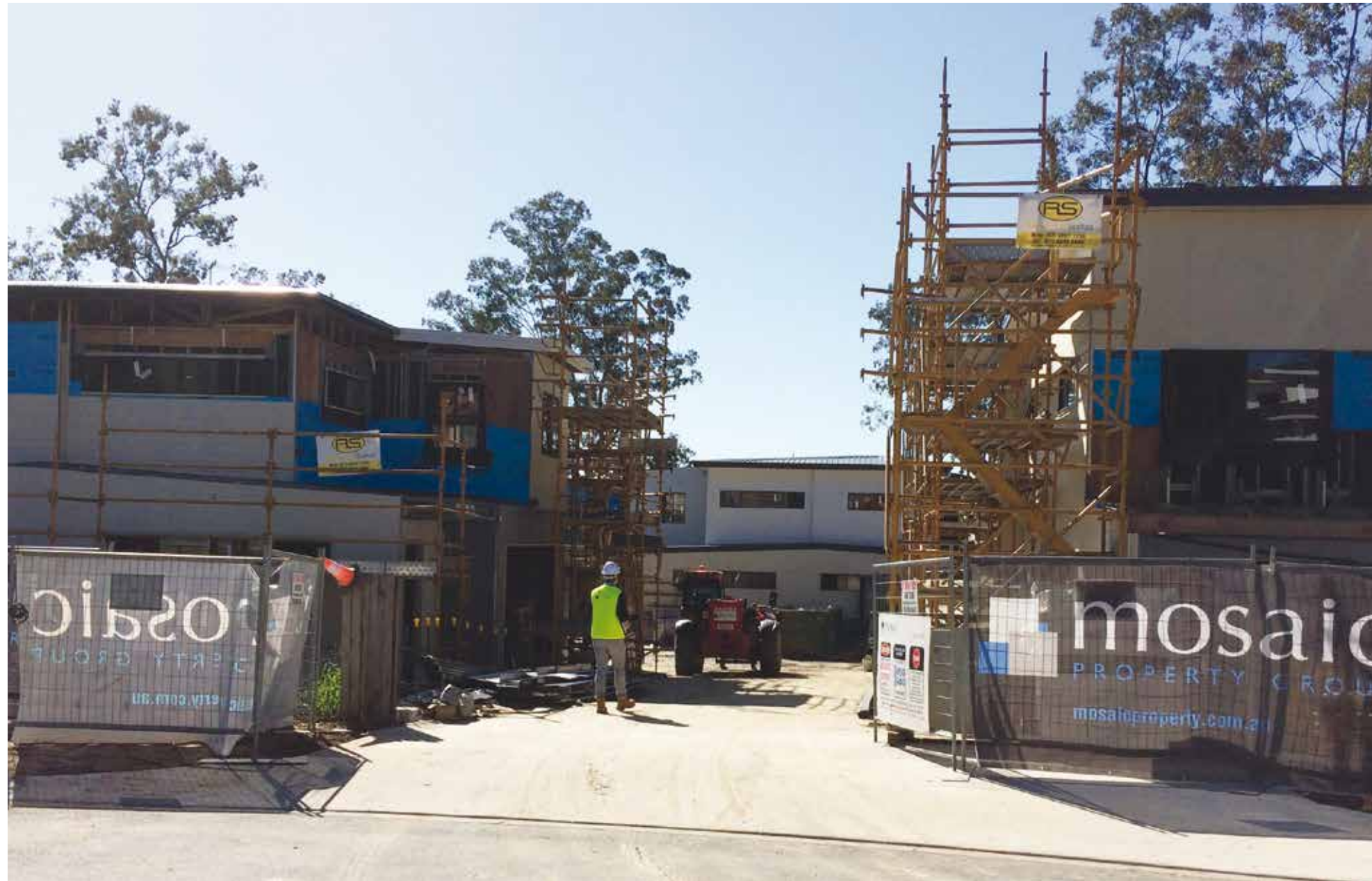
Town houses 1 – 7 had windows installed as well as the structural steel on the back decks, with town houses 3 – 10 also having external sheeting and cladding fitted. With town houses 12 – 21 being more advanced, work was focused on the internals, including tiling, sheeting and painting.
