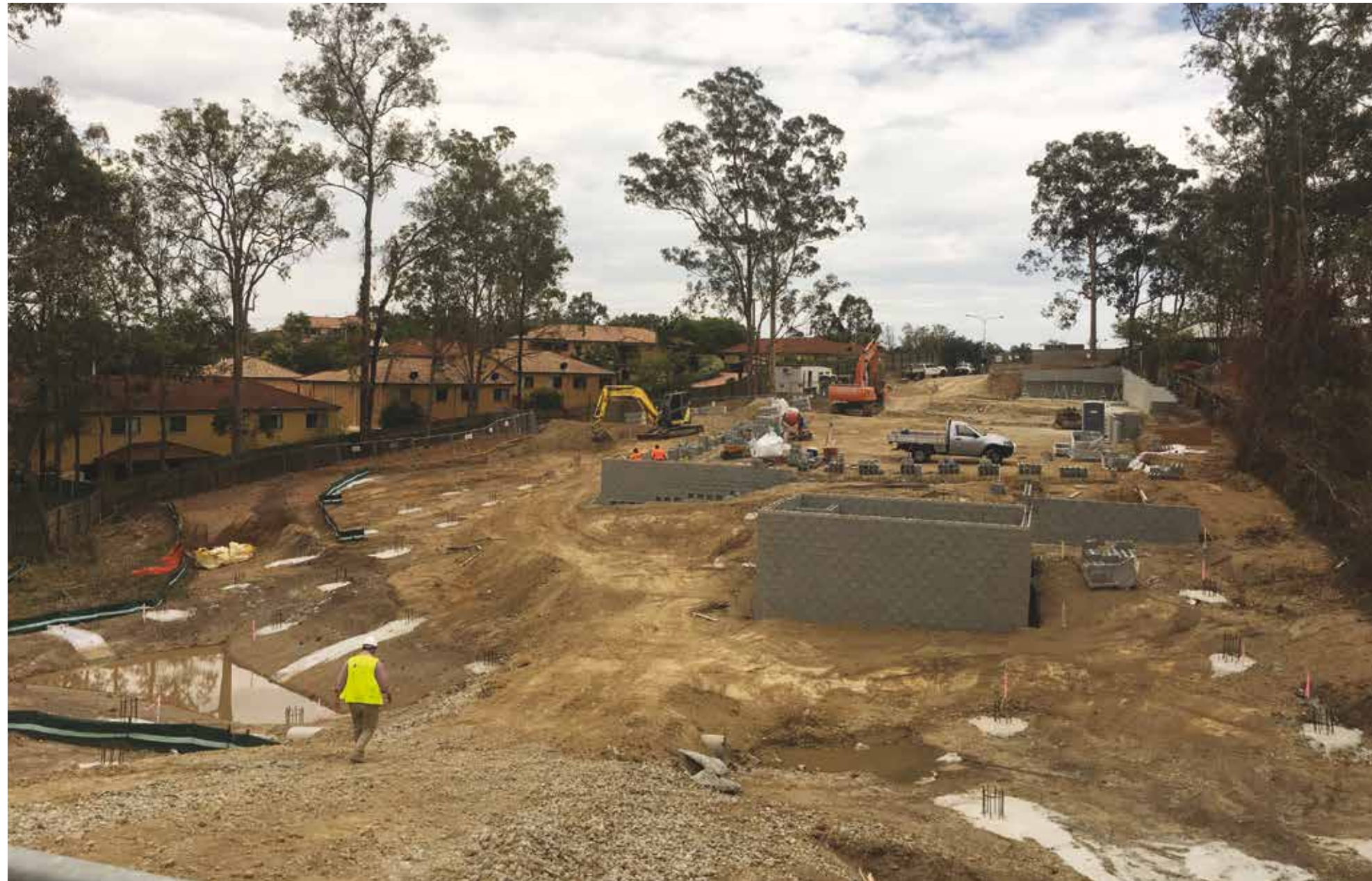
Detailed excavation is underway for town houses 7 – 10, with building pads now cut and formed. Blockwork has started, with the retaining wall for the southern boundary laid, backfilled with concrete and waterproofed.
