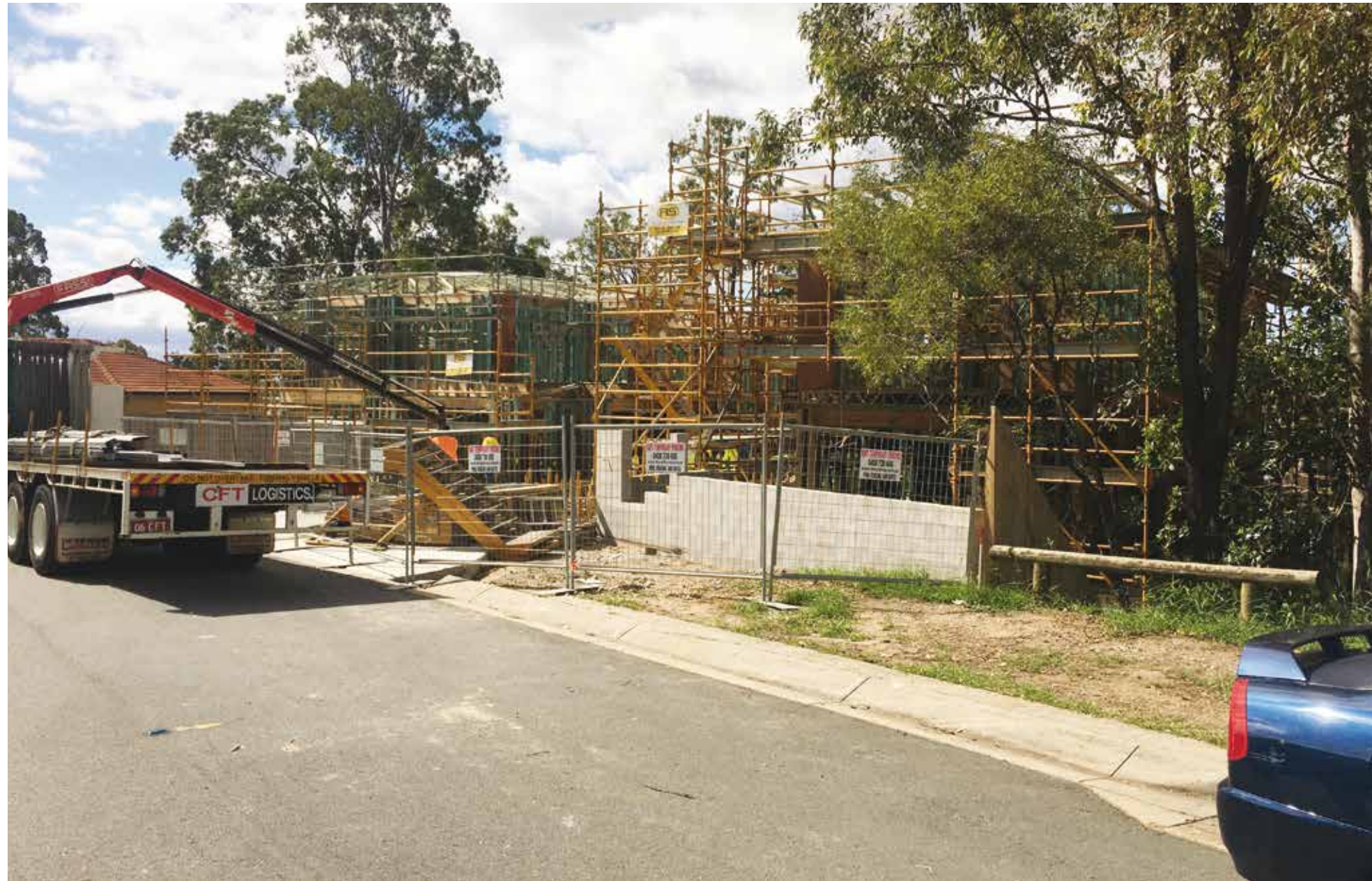
The building pad was cut and under slab draining installed in town house 11, while cladding is nearing completion on town houses 12 – 18. Internal wall and ceiling sheets were installed and sanded, enabling painting to commence.
