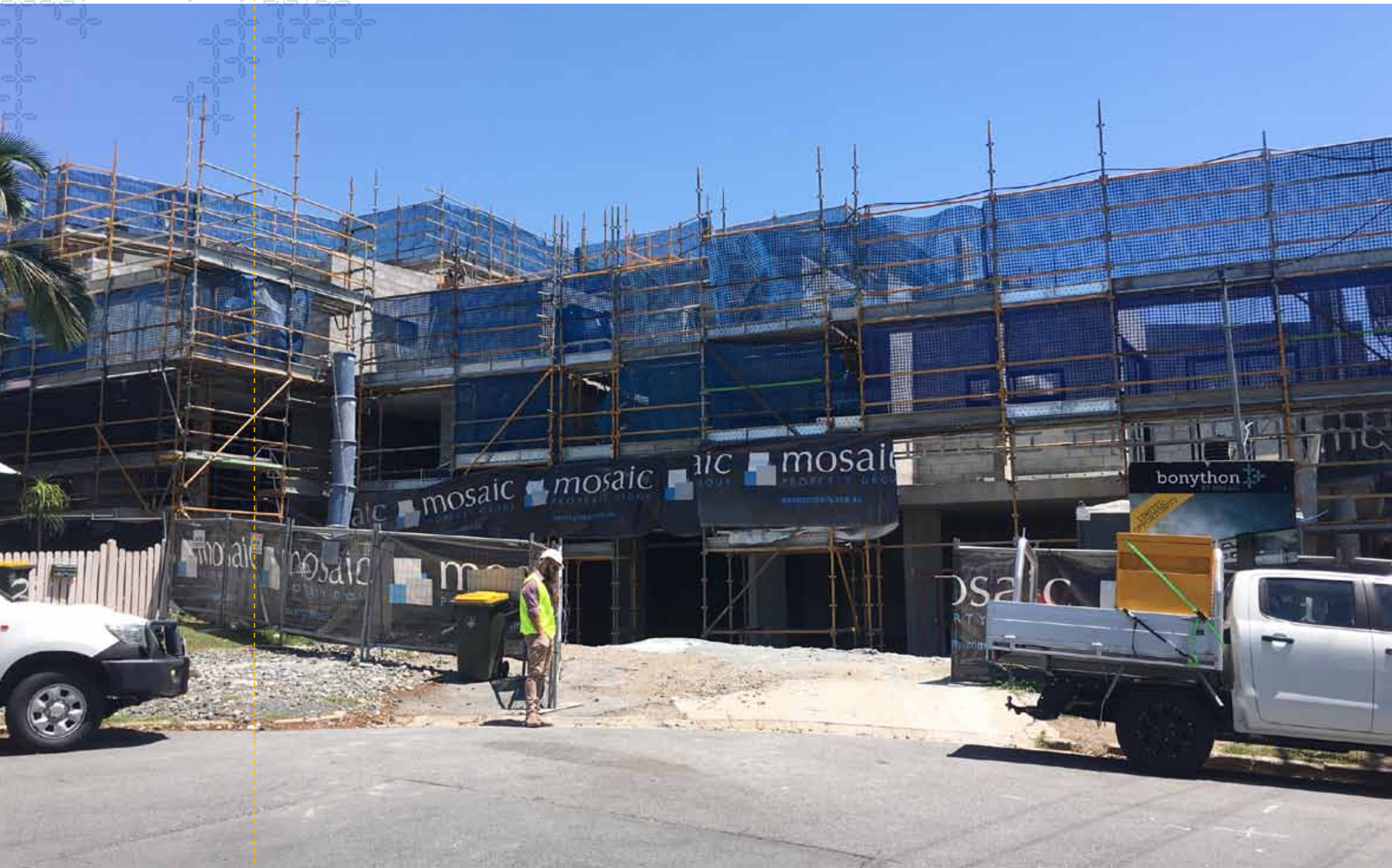
The complex nature of the roof structure resulted in some delays, however the development continued to take shape internally and externally.
