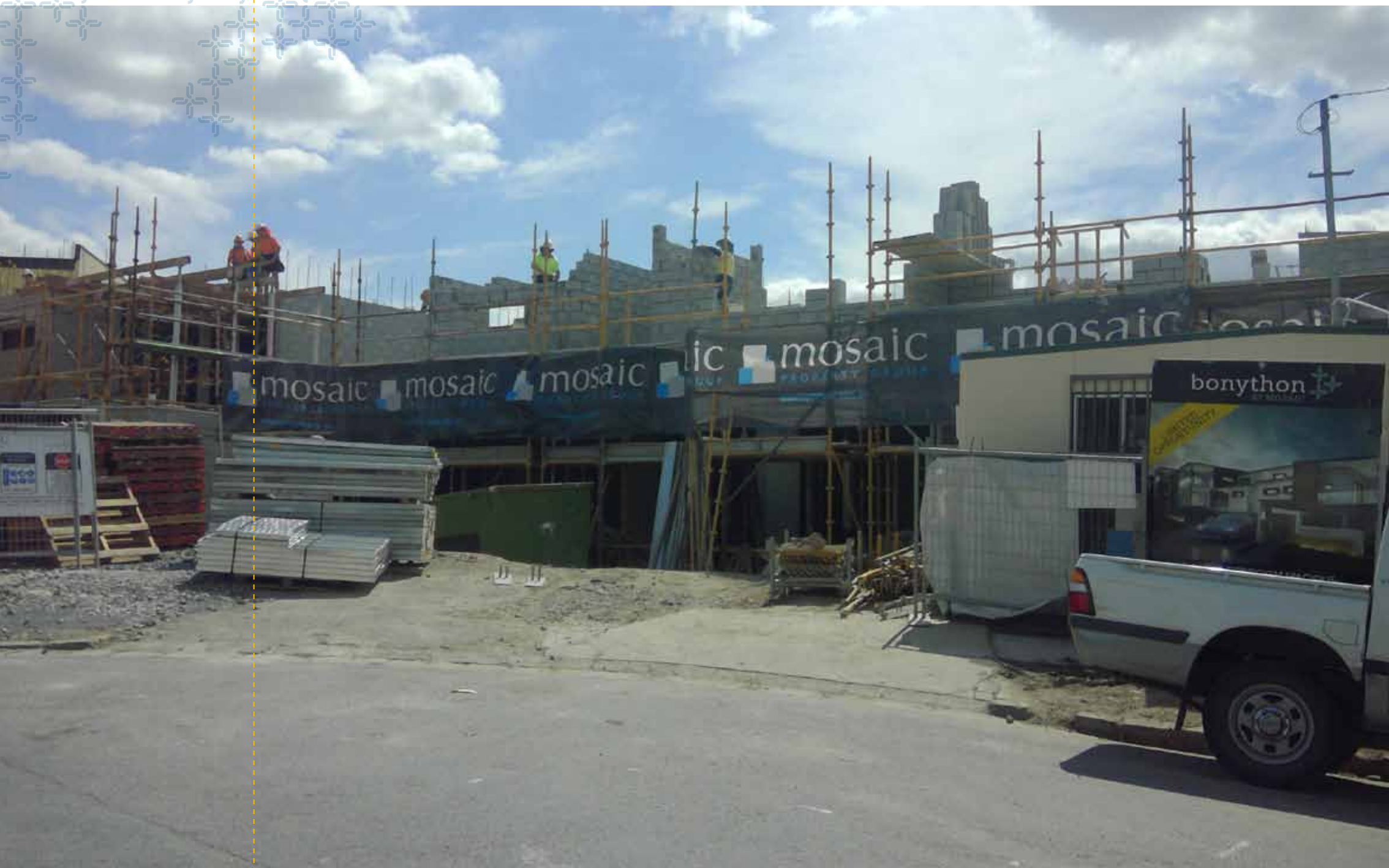
650m 3 of concrete was poured to create the Level 2 slab. Backfilling of the voids between the Level 1 external walls and the northern property boundary were also completed.
