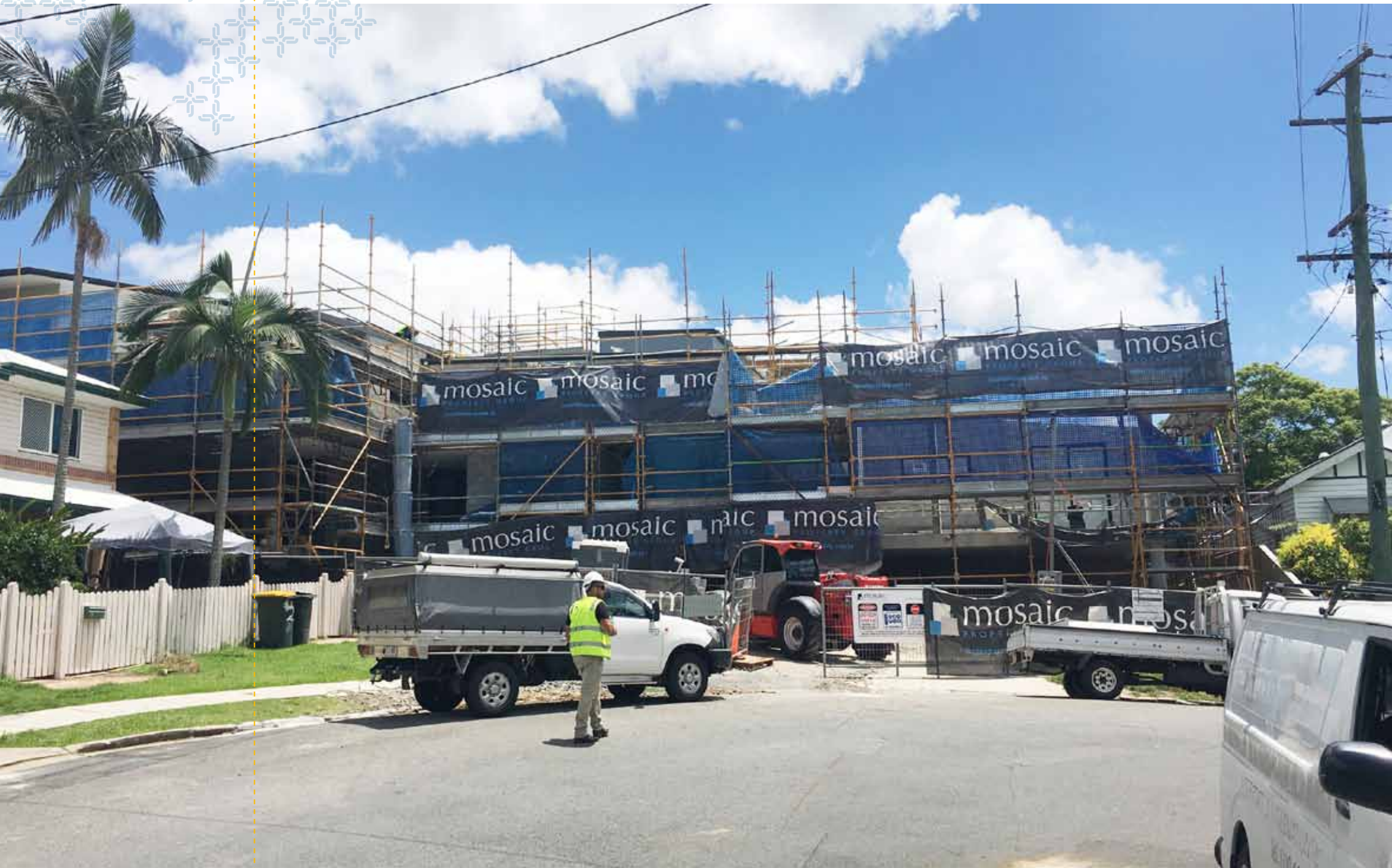
As the scaffold started to come down, the first glimpse of the top floor was visible from Bonython Street.
