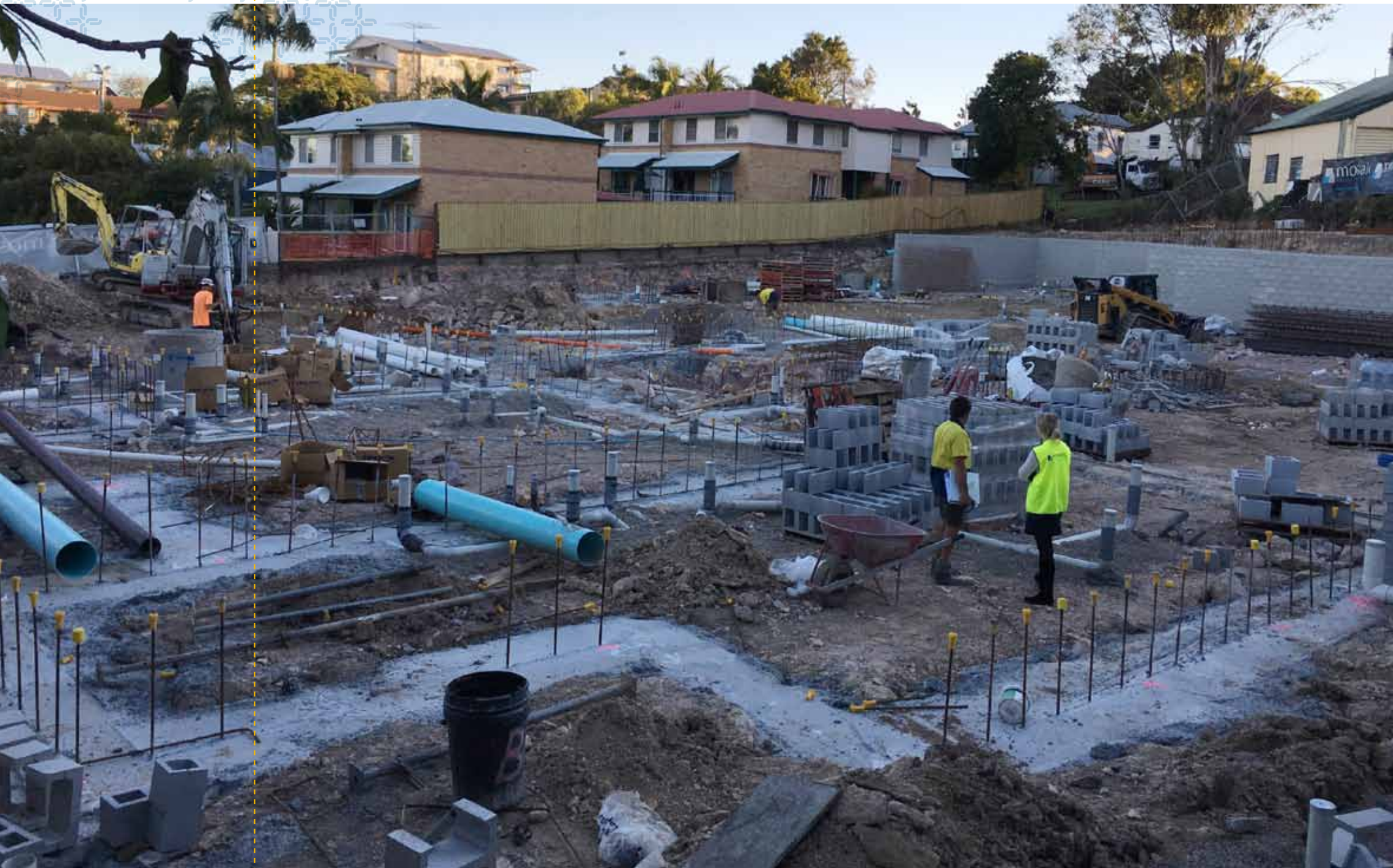
Noticeable progress on site with the completion of bulk earthworks. Excavation reached the required depth for the car park and Level 1 slab and the concrete footings were poured, creating a level base for the installation of core-filled blockwork retaining walls.
