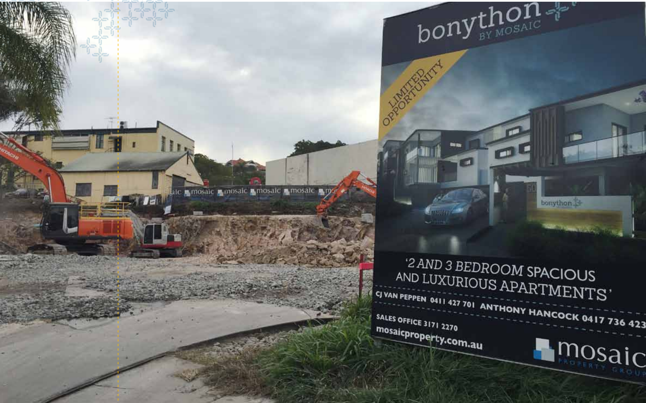
The first month was quite challenging with the construction team encountering some very tough ground conditions. Bulk excavations commenced with trucks on a continual turnaround removing 5,500m 3 of material using a 35-tonne excavator.
