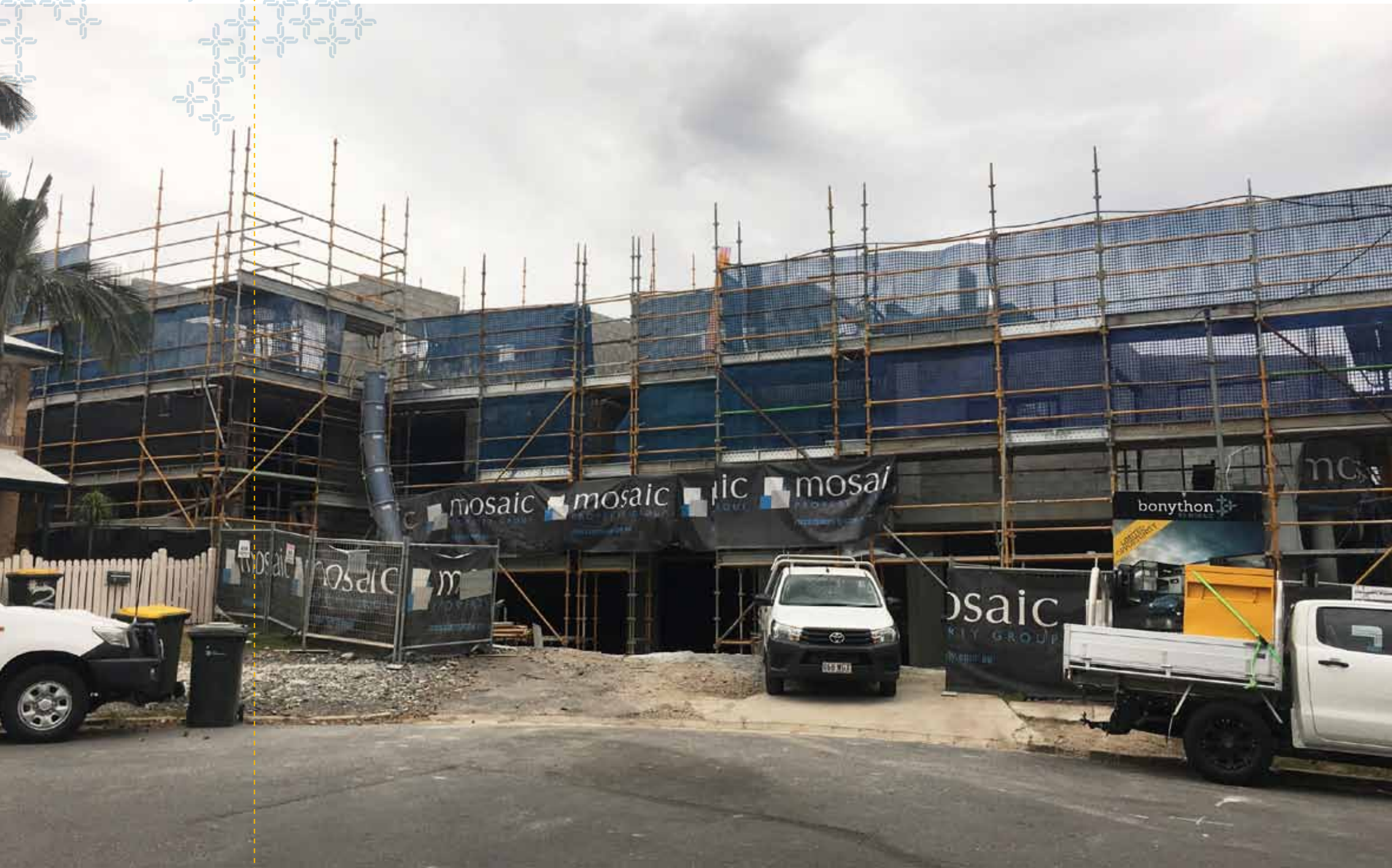
The building steadily moved upwards as the Level 4 slab was poured. Internally, Level 1 apartments were sheeted and set with windows and door frames installed.
