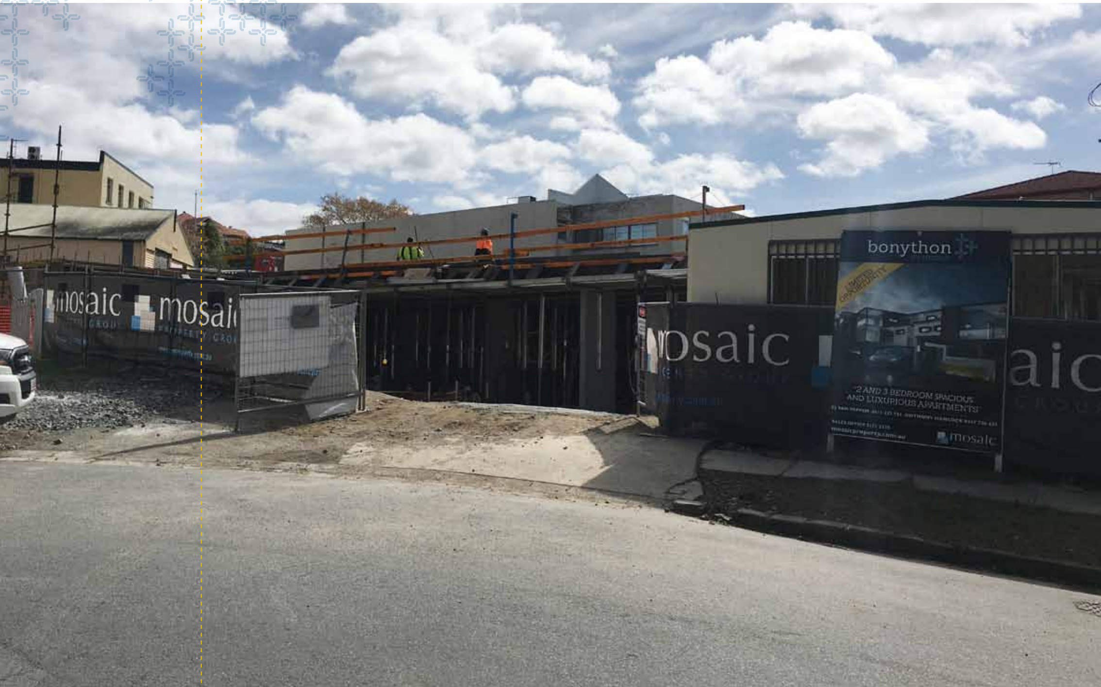
Bonython started its vertical ascent as the build gathered pace. Stormwater connections were installed and the car park and Level 1 slabs finished, taking over 1,200 square metres of concrete.
