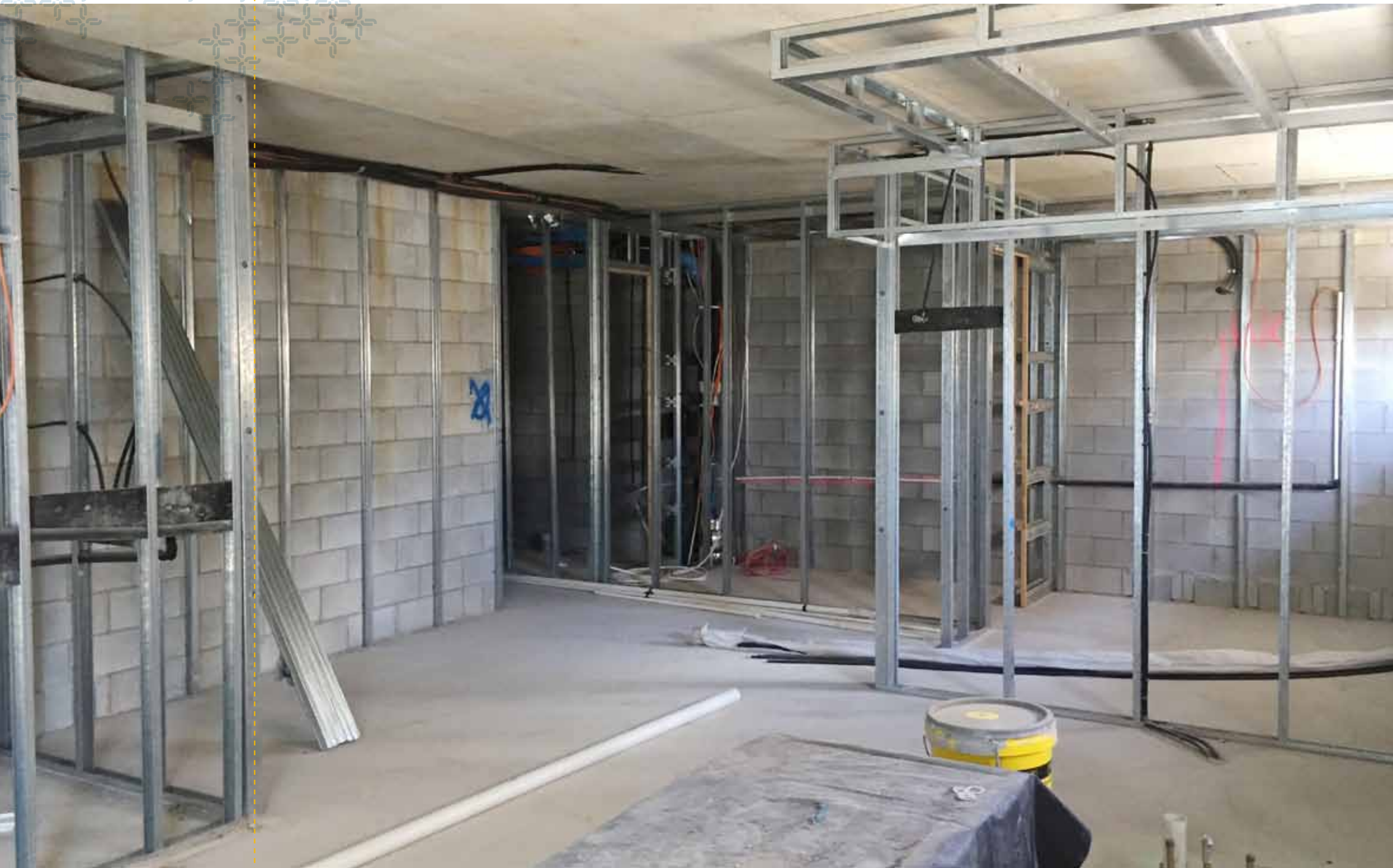
It was all hands on deck as the development moved into the final stages, with approximately 75% of the rendering, cladding and painting as well as most of the apartments across Levels 1 to 3 completed.
