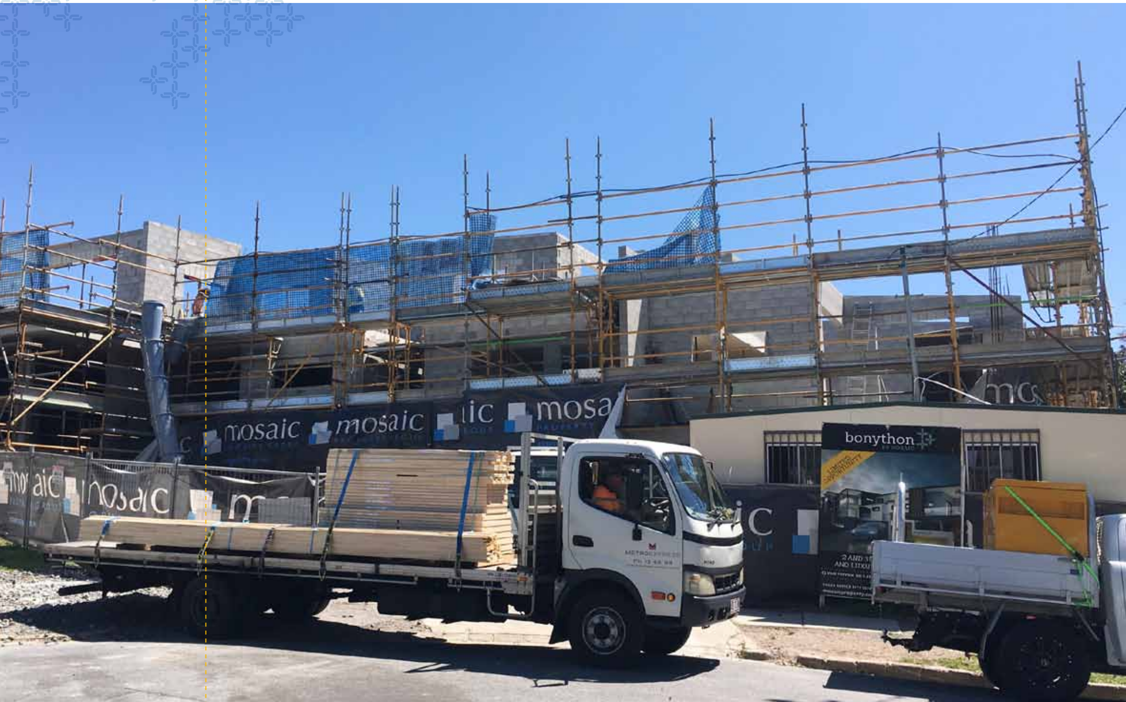
City views continued to unfold as Bonython reached Level 3, where the slab was poured and cured, allowing the core-filled blockwork to be laid to the underside of Level 4.
