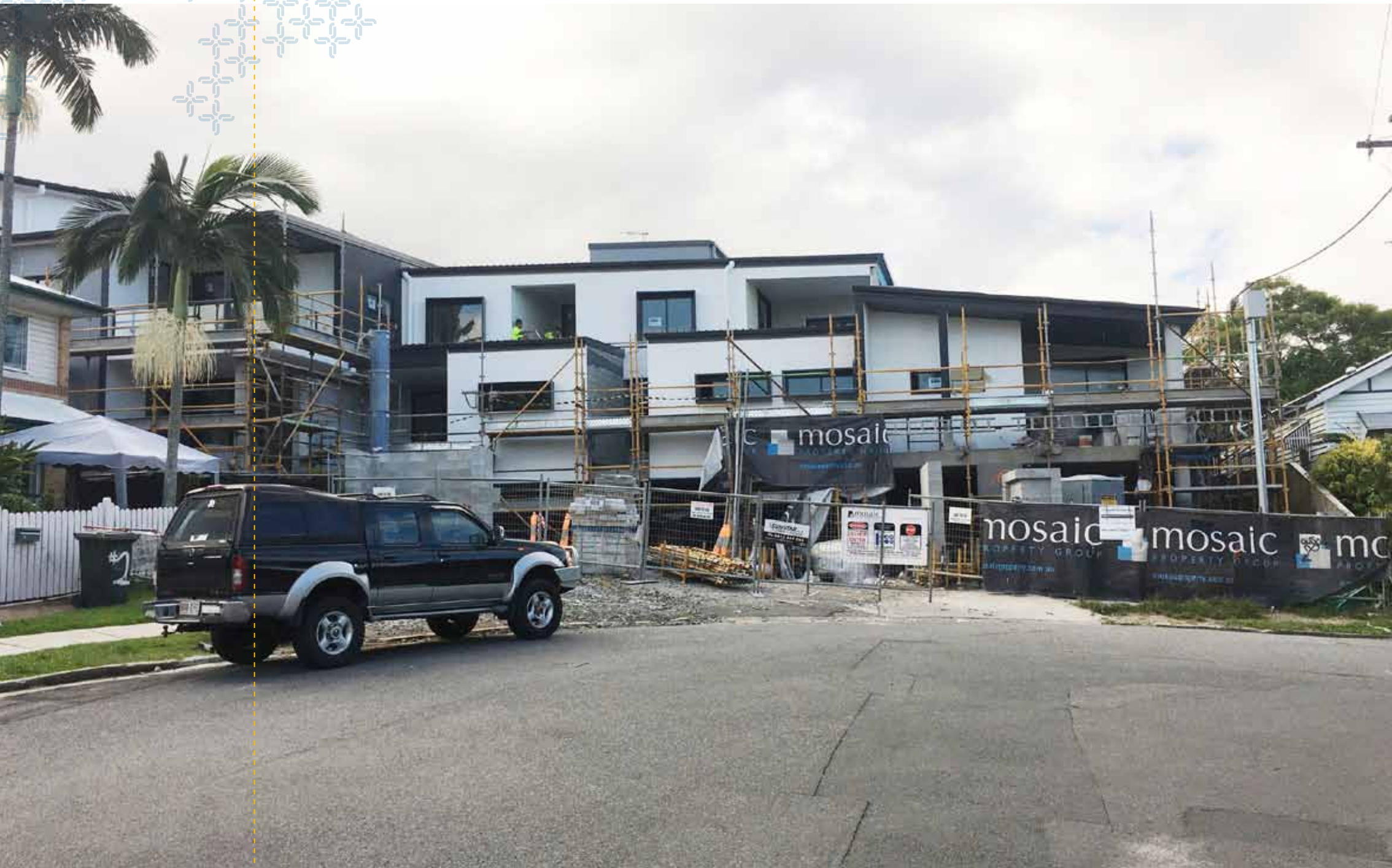
With the majority of the scaffold stripped from the external façade, the stylish and clean building architecture was fully exposed. Internally, substantial progress.
