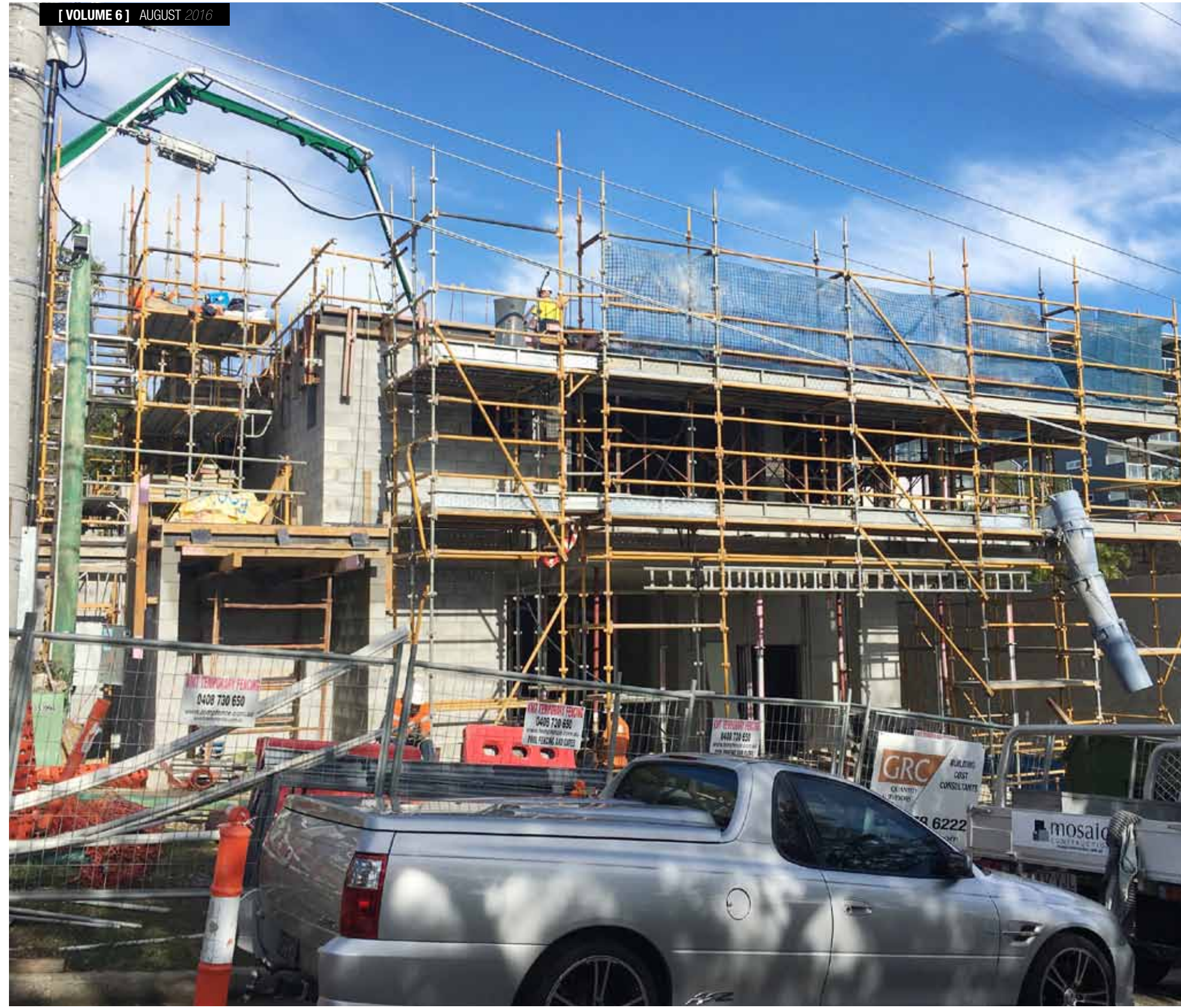
With the Level 1 structural columns formed and poured, core-filled blockwork walls were laid and run up to the underside of Level 2.
