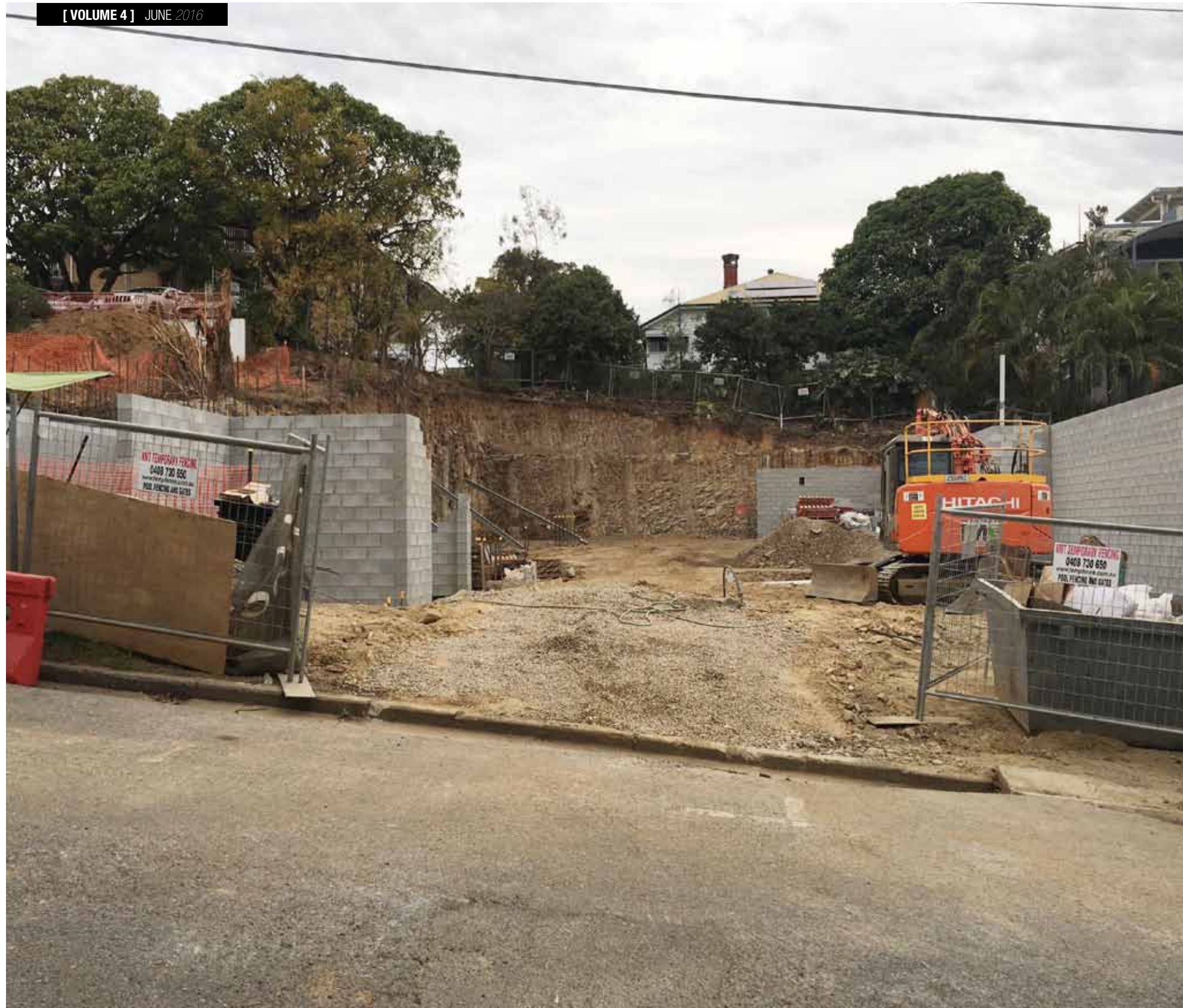
The vertical cut face was excavated back to expose the bored piers, which allowed the retaining wall footings to be excavated before reinforcement was placed and concrete poured.
