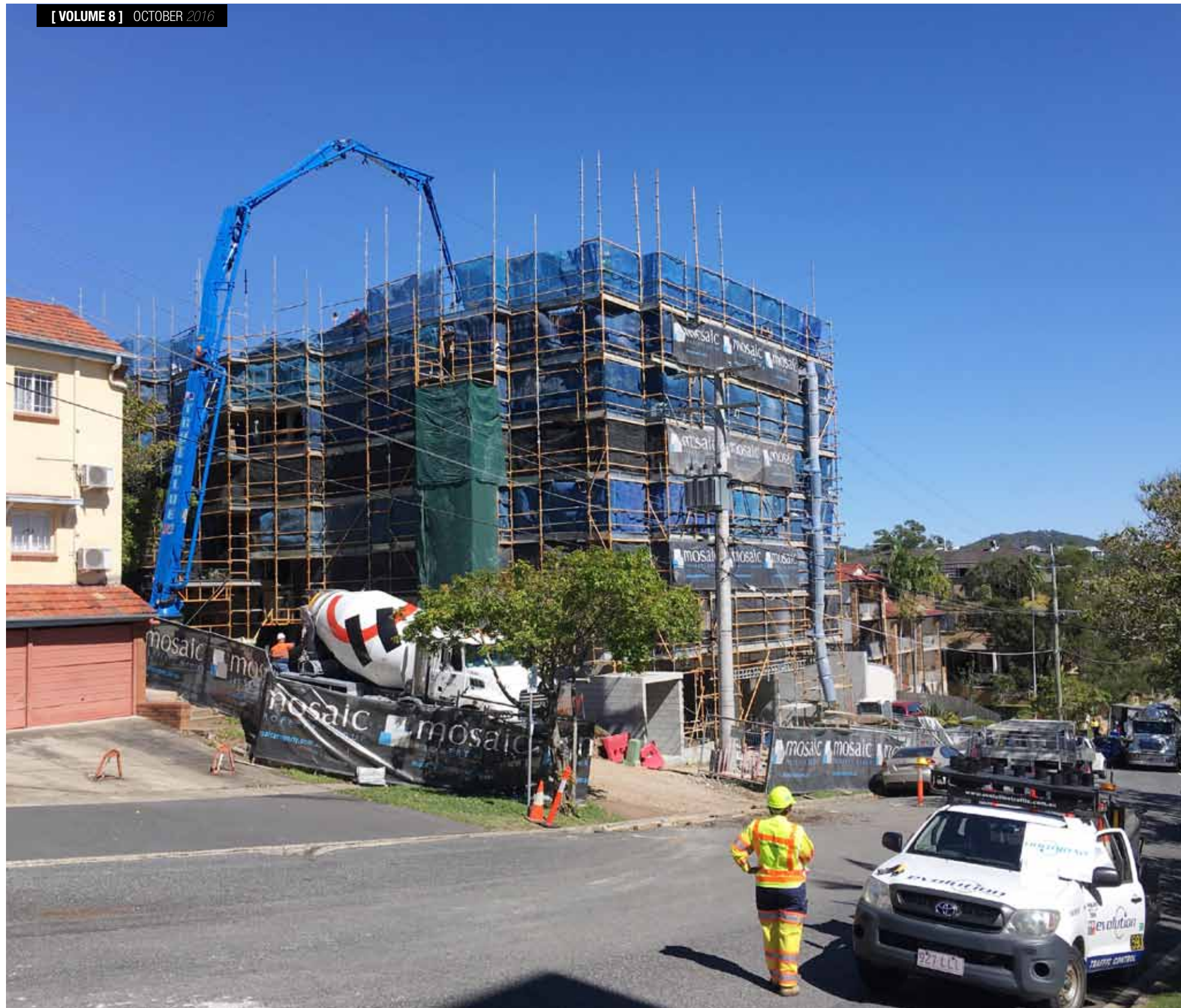
The formwork deck and back-propping system for the Level 4 slab were installed, conduits run and reinforcement mats fixed into position before pouring the concrete.
