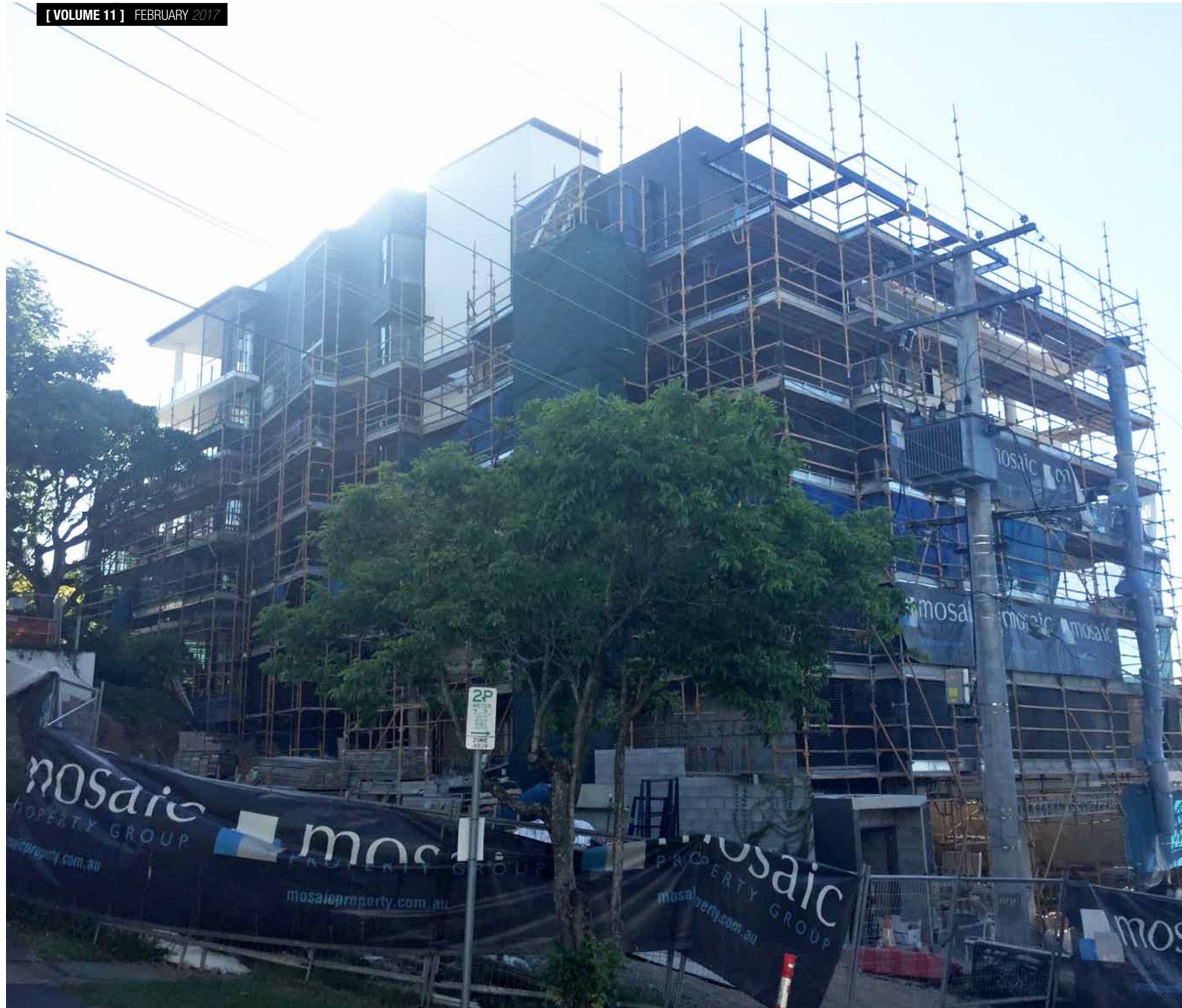
The external facade is becoming further exposed as the scaffolding is stripped from Level 6 down to Level 4. Internally, substantial progress.....
