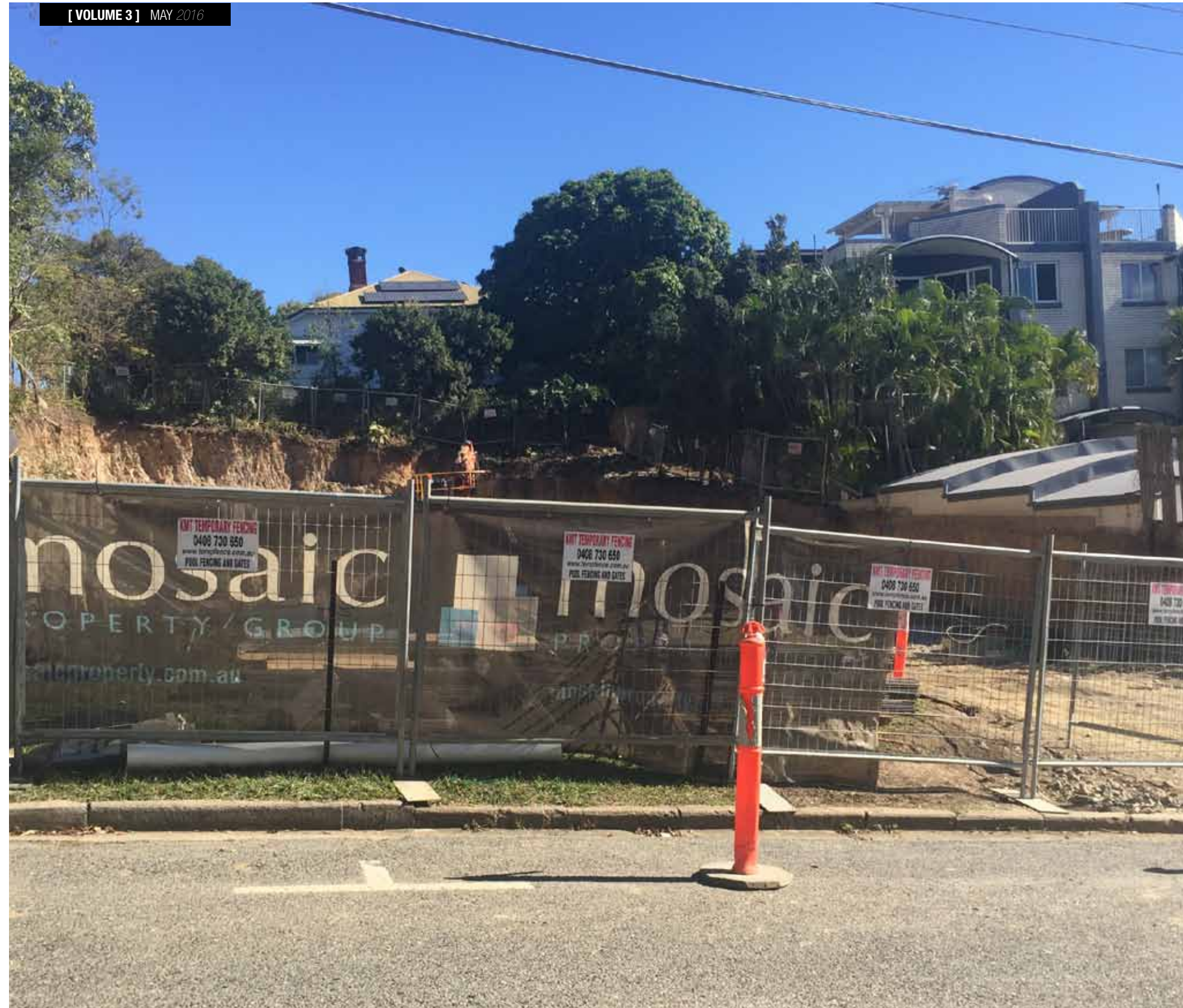
Excavation for the foundations of the required structural retaining wall and columns of the building are nearing completion, with reo cages installed and concrete poured, leaving the column starter bars exposed.
