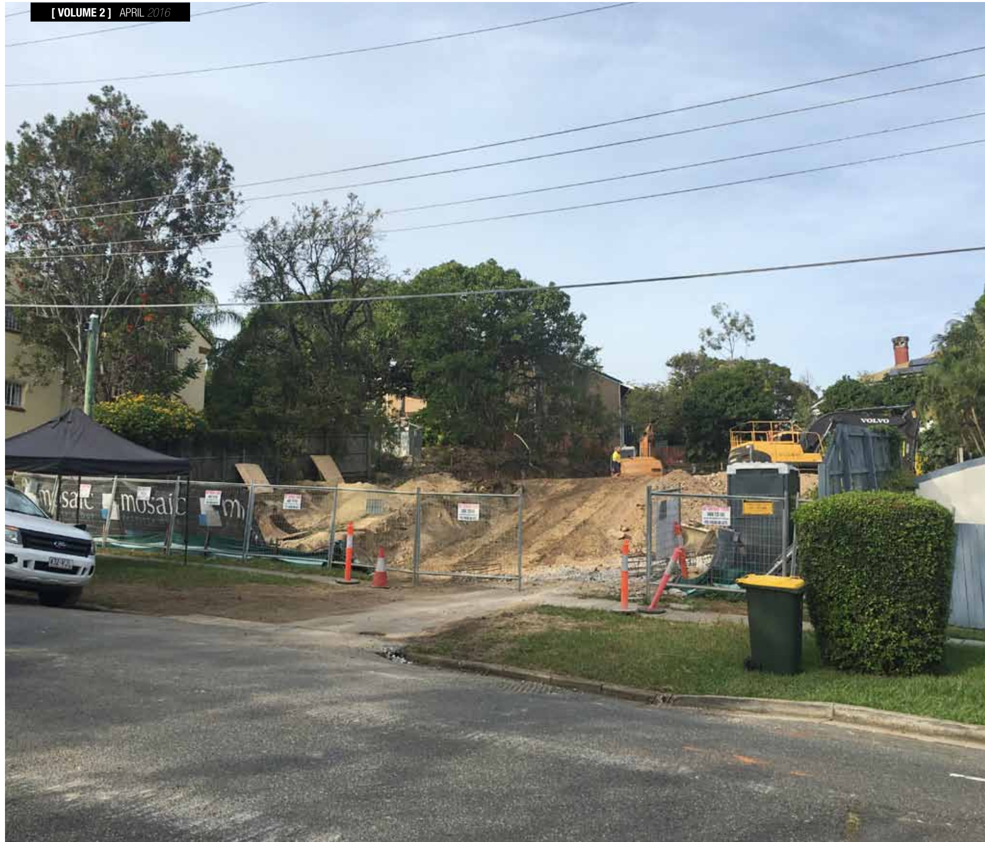
Although detailed geotechnical investigations undertaken on the site had identified some sub-surface rock, once the drilling commenced we found that the rock shelf was larger than originally anticipated, so the drilling took slightly longer than allowed for in the program.
