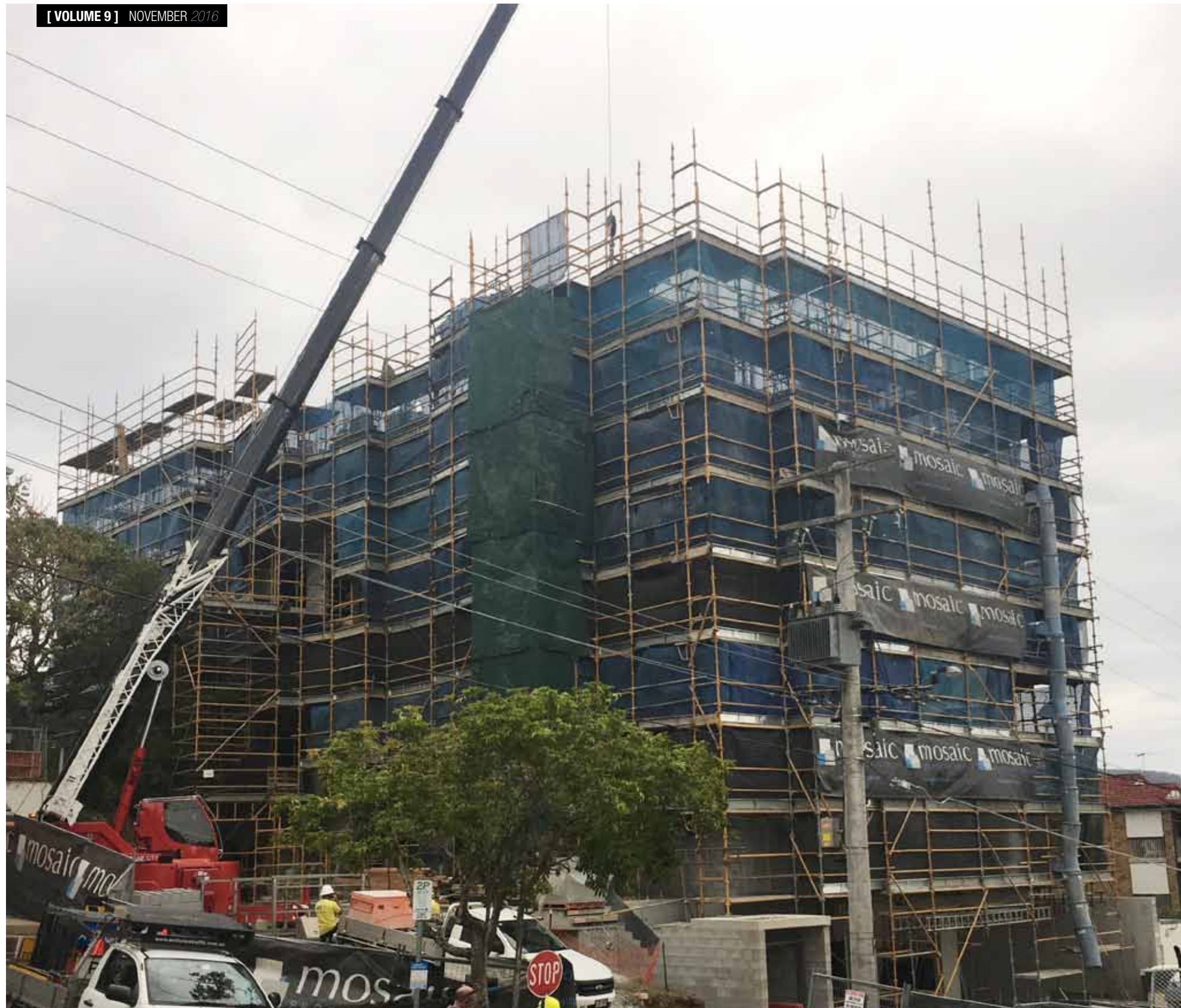
With two slabs poured over the course of the last month, Arc on Lima continues to show strong progress as it steadily moves upwards.
