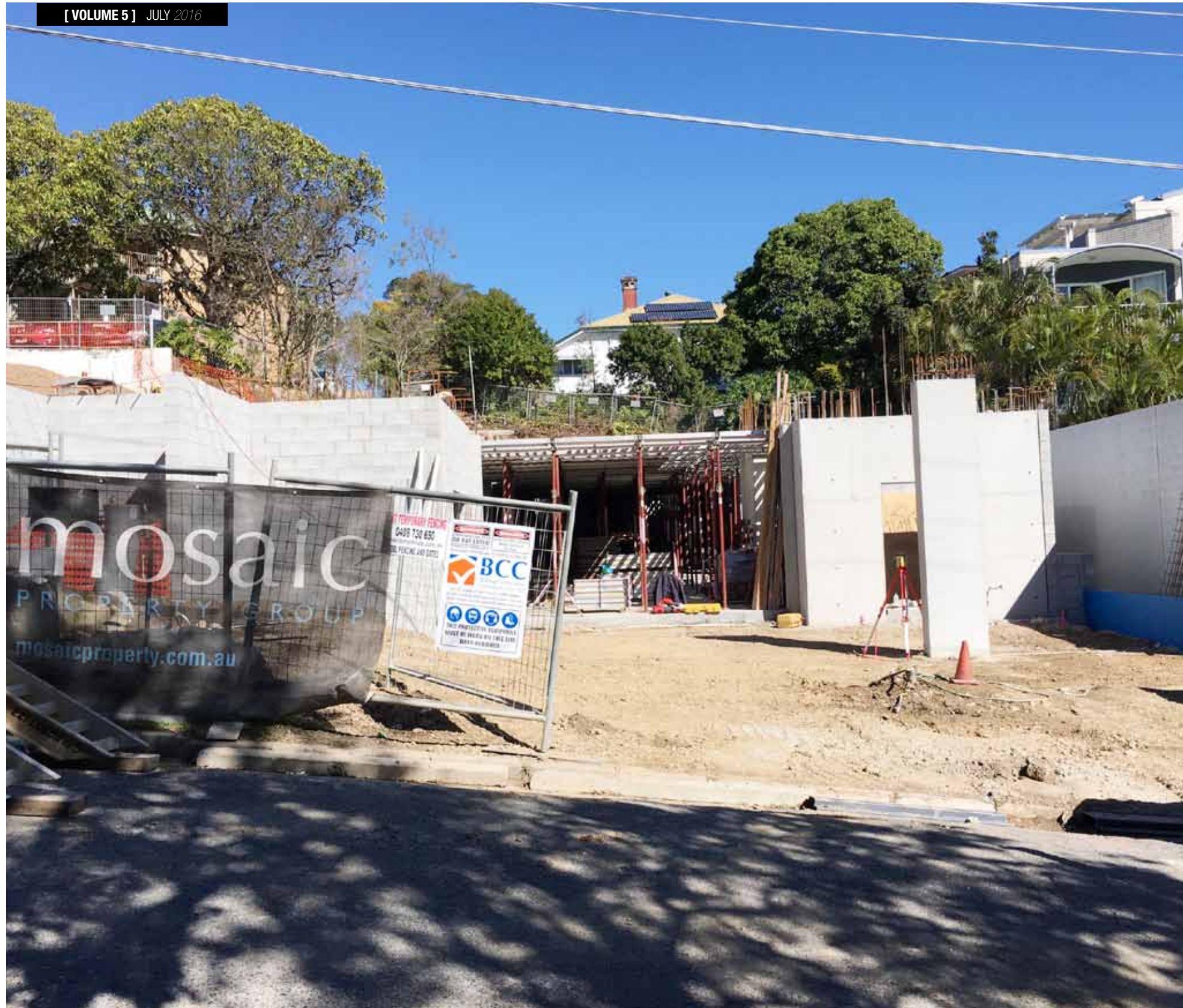
The core-filled blockwork retaining wall around the perimeter of the site was installed and waterproofed, while structural columns to the underside of Level 1 were formed, reinforced and poured.
