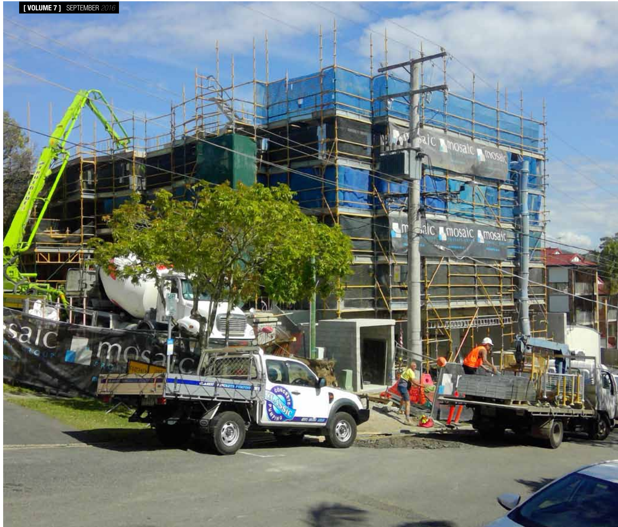
After the Level 2 slab was poured and reached maximum strength, blockwork walls were run to the underside of Level 3 and structural columns were formed and poured.
